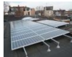
Mercury Solar A commercial solar-power system installed by Mercury Solar in Pennsylvania.
