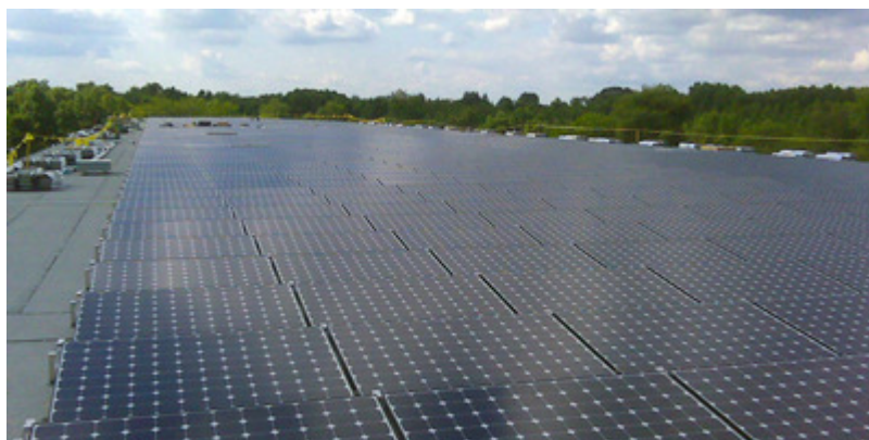
Figure 1: A 383 kW commercial installation in Deptford, NJ, Courtesy of Mercury Solar Systems
